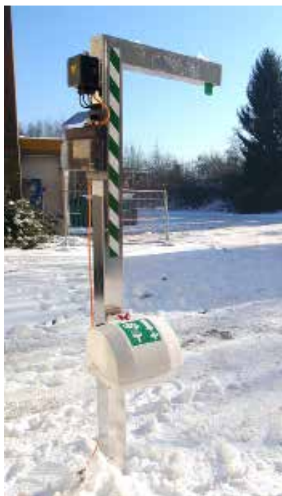
Nooddouche in wintermodus / Safety shower in wintertime
